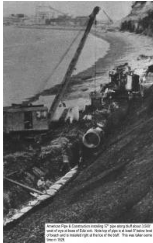
Figure 4. 1929 installation of Elwha industrial pipeline at the base of Elwha feeder bluffs. Subsequent armoring have resulted in severe sediment starvation along the Elwha nearshore. Photo provided by Dean Reed, Nippon Paper Company
